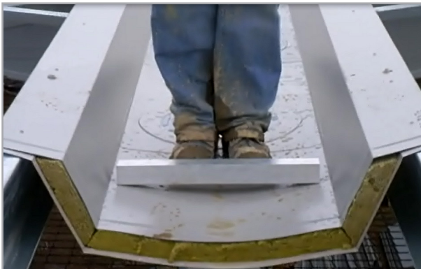
Thin gauge steel and the deflection
