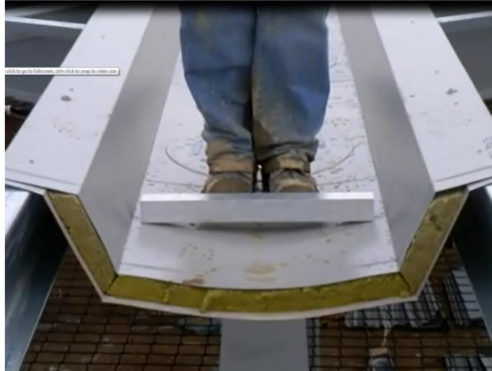
Thin gauge steel and the deflection
